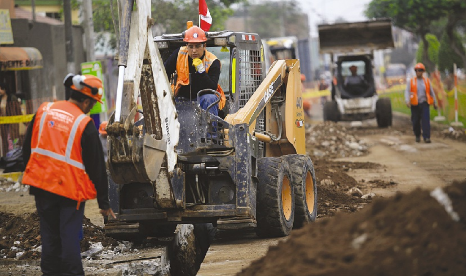
Men at work: the installation of natural gas pipelines in capital Lima is evidence of Peru's attempts to fill the infrastructure gap
